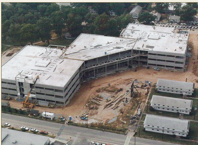
U.S. Army Forces Command Headquarters (Command and Control Facility, Marshall Hall) Under Construction, 1985.
